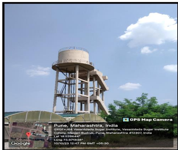
Water tank (Capacity: 1 lakh litre)
