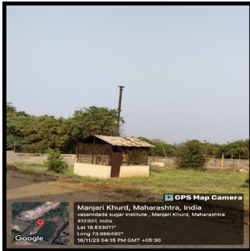
Incinerator installed for solid waste
