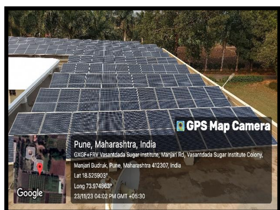
Solar Plant installed
